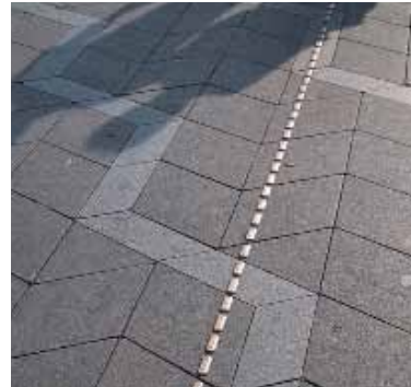
High quality paving with 'lines' to orientation for blind people. Copenhagen, Denmark
