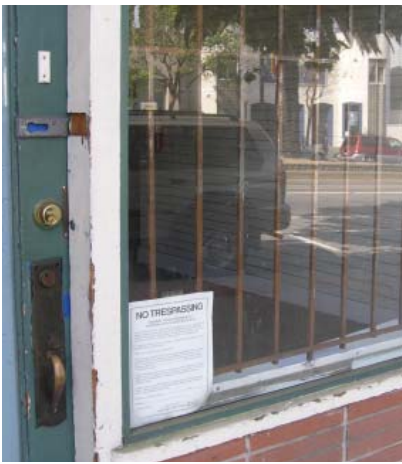
Empty storefront in need of facade improvement
