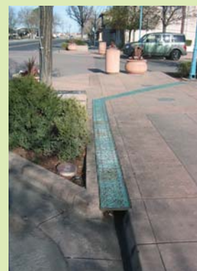
Trench drains may be used to allow pre-existing catch basin locations to be maintained and decrease the potential cost of curb extension construction. See Section 6.2 for appropriate use and design of trench drains.
